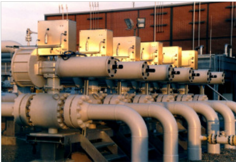
Manifold of the gas injection and withdrawal plant at surface.
