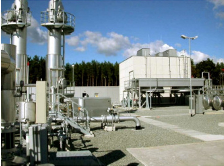
Surface plant of the underground storage facility Peckensen with gas dehydration units
