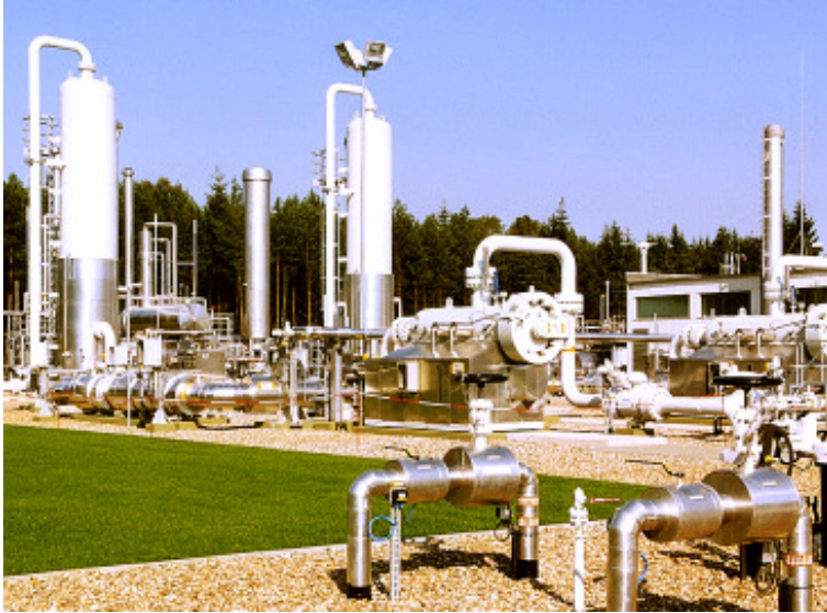
Surface plant of the underground storage facility Kraak - Filters and dehydration plants
